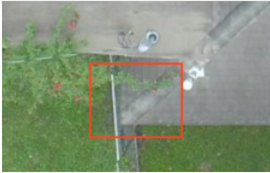
1035724 Severity: 4 Worn section
