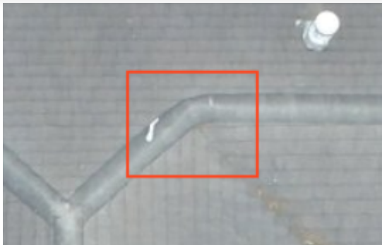
1035725 Severity: 4 Worn section
