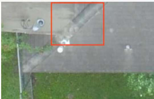
1035726 Severity: 4 Worn section
