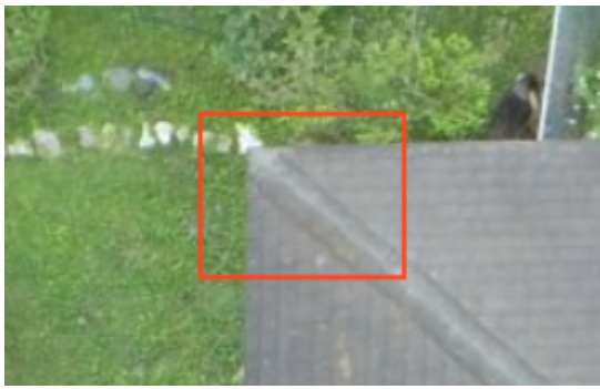
1035722 Severity: 4 Worn section
