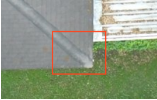
1035723 Severity: 4 Worn section
